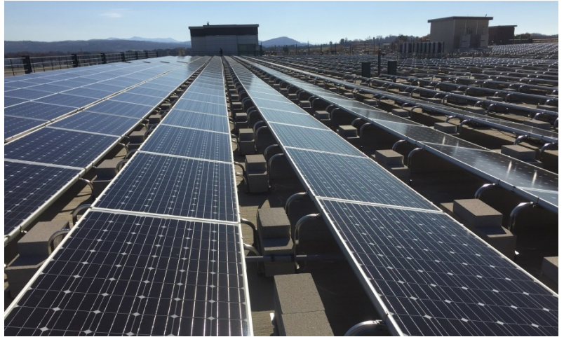
BED solar array at Burlington International Airport
